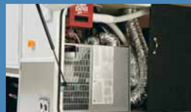
A sliding door provides handy access to the furnace, central vacuum and other mechanic items.
