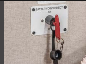
Exterior Battery Disconnect A turn of the knob keeps your battery from discharging.
