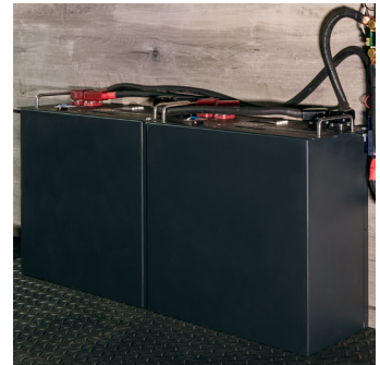
(2) 200AH 48V Lithium Batteries (which is equal to (8) 100AH 12V Lithium Batteries)*
