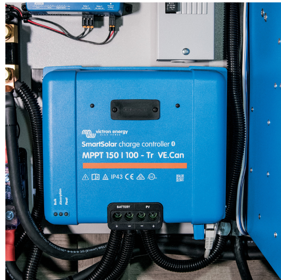
100 amp Victron MPPT Solar Charge Controller
