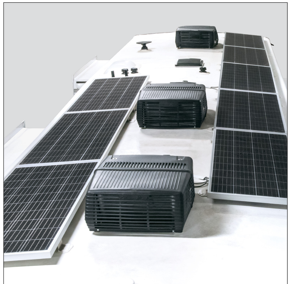
(8) 220W solar panels = 1,760 Watts of solar power
